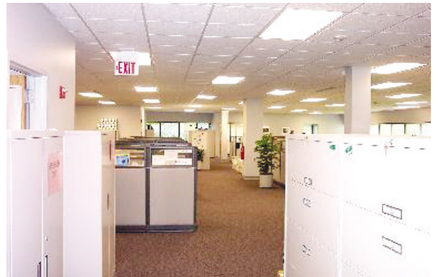
CI Select installed 150 i-ceilings Privacy speakers at this call center to help SSM Health Care comply with HIPAA regulations in this sensitive area.
